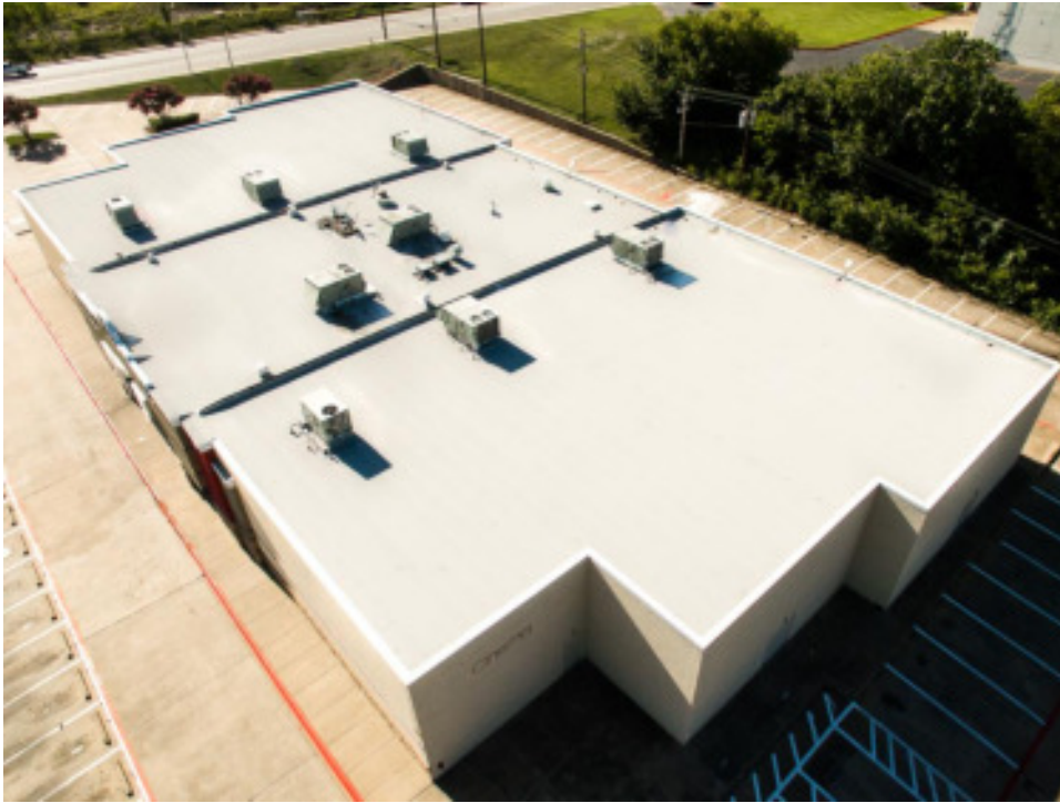
Low-slope roofing membrane installed using a propane torch and consisting of a SBS-modified bitumen cap sheet and base sheet.
