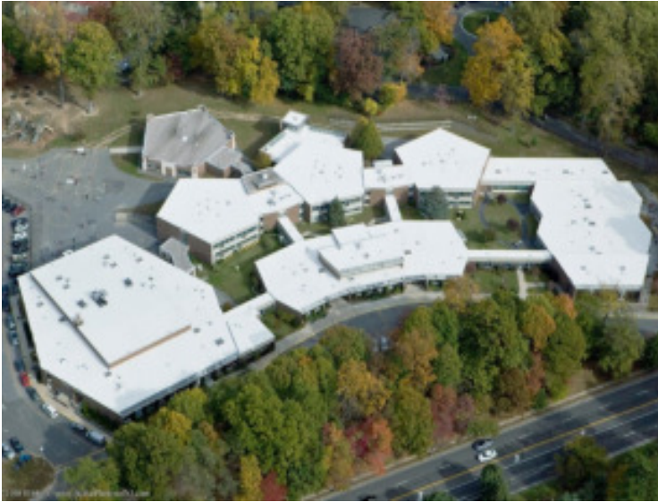
Low-slope roofing membrane installed using low-VOC adhesive and consisting of a SBS-modified bitumen cap sheet and base sheet.
