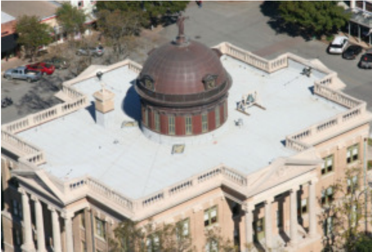
Low-slope roofing membrane installed using a propane torch and consisting of an APP-modified bitumen cap sheet and base sheet.
