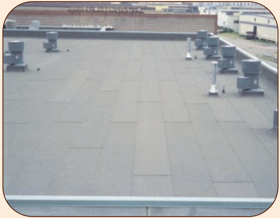
For this roof system, the base sheet and ply sheets, as well as the modified bitumen cap sheet, were applied in hot asphalt. Photo courtesy of CertainTeed Corp., Valley Forge, Pa.
