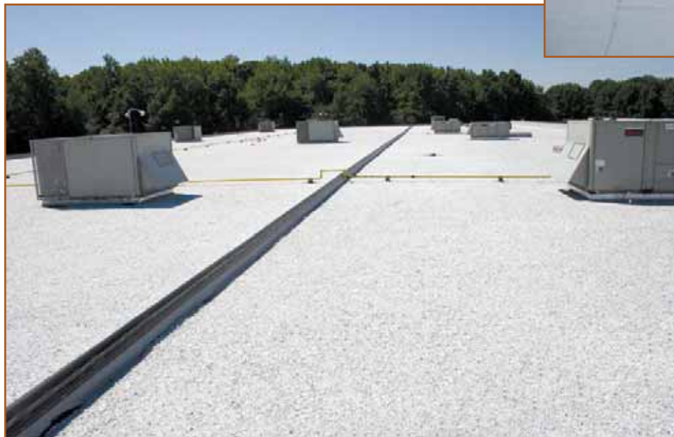
Left – A traditional built-up roof (BUR) covers this laboratory building. BUR is one of the longest-lasting roofing systems available. (Photo courtesy of GAF, an ARMA member.)
